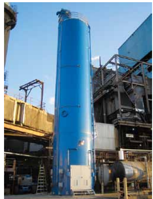
Silo based equipment for B-PAC injection
